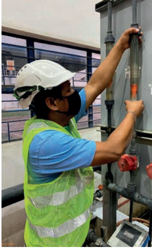
Employees ensured around the clock water availability at a minimum of 7 psi.
