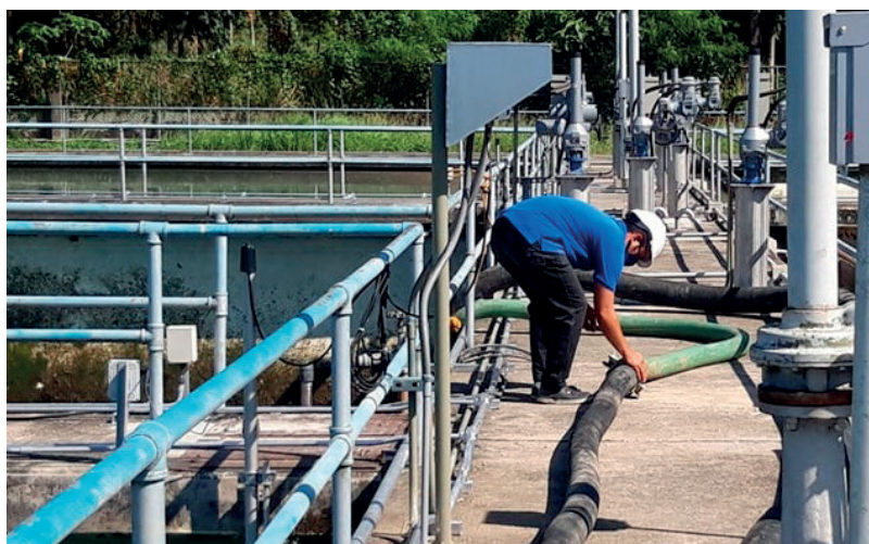
Manila Water continued to improve its facilities despite the pandemic, investing ₱12.1 billion in capital expenditures in the year.
