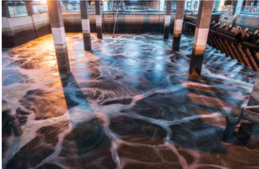
Apart from providing clean and potable water, Manila Water also provides sewage and sanitation services.
