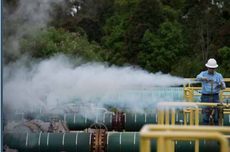
In April 2017, as part of a consortium, AC Energy completed its acquisition of Chevron's assets in Indonesia, including the Salak and Darajat geothermal fields in West Java.
