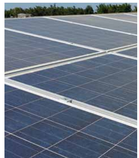
The San Carlos Solar farm is one of AC Energy's three solar farms in the Visayas.
