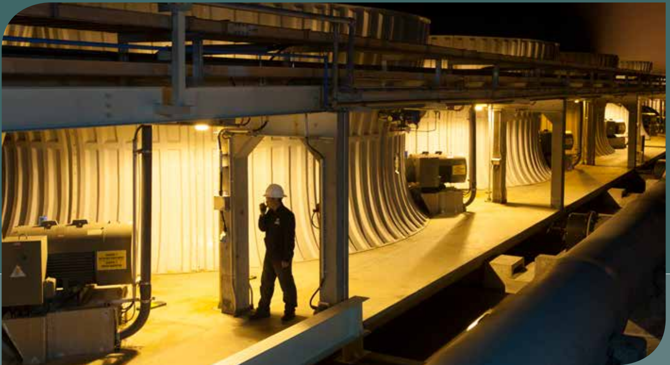
The Salak and Darajat geothermal plants in Indonesia contributed to AC Energy's equity earnings beginning in April 2017.
