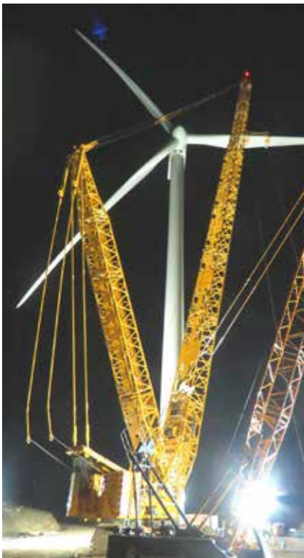
Once completed, the Sidrap project will be Indonesia's first utility scale wind farm.
