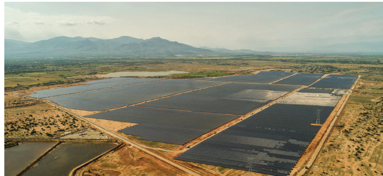
AC Energy 330 MW Ninh Thuan solar farm in Vietnam is one of Southeast Asia's largest solar farms.
