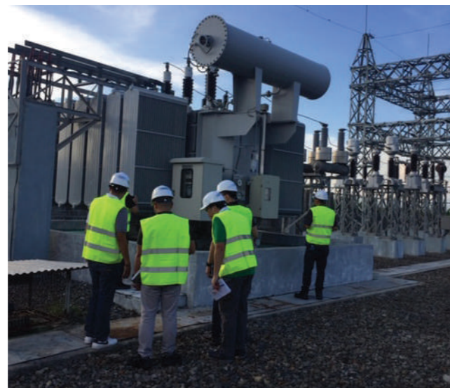
Risk Engineering Survey conducted by AON and insurers for our solar plants.
