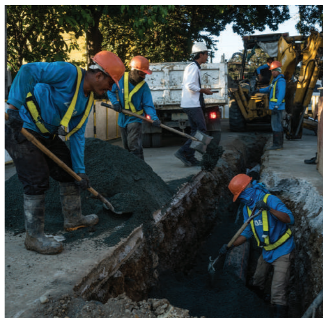
Manila Water's pipelaying activities ensure efficient water distribution in all its serviced areas.
