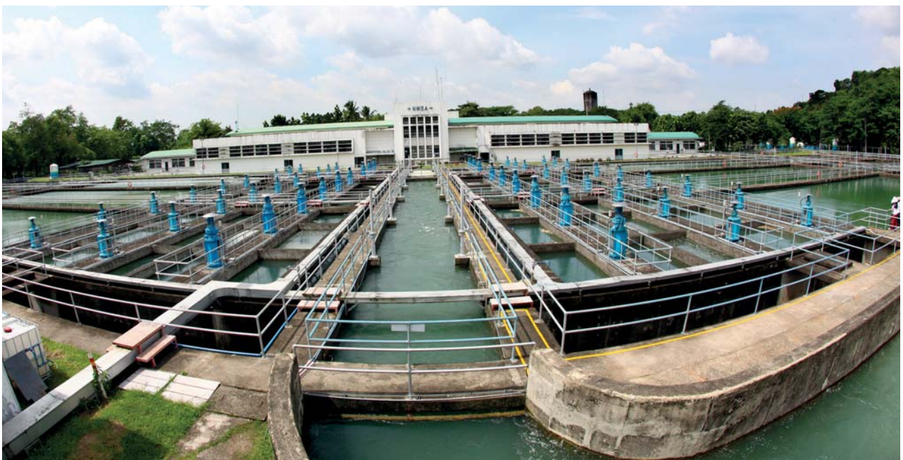
Manila Water continues to invest in infrastructure in order to ensure the highest quality of its services.
