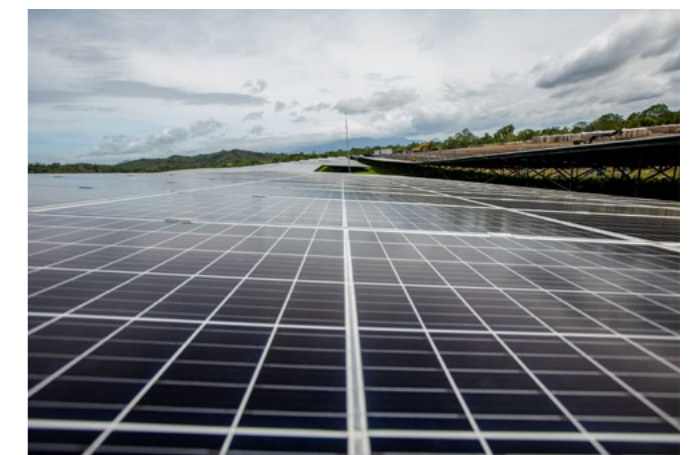
ACEN's Alaminos Solar Farm in Laguna supplies renewable energy to customers seeking to reduce Scope 2 GHG emissions
