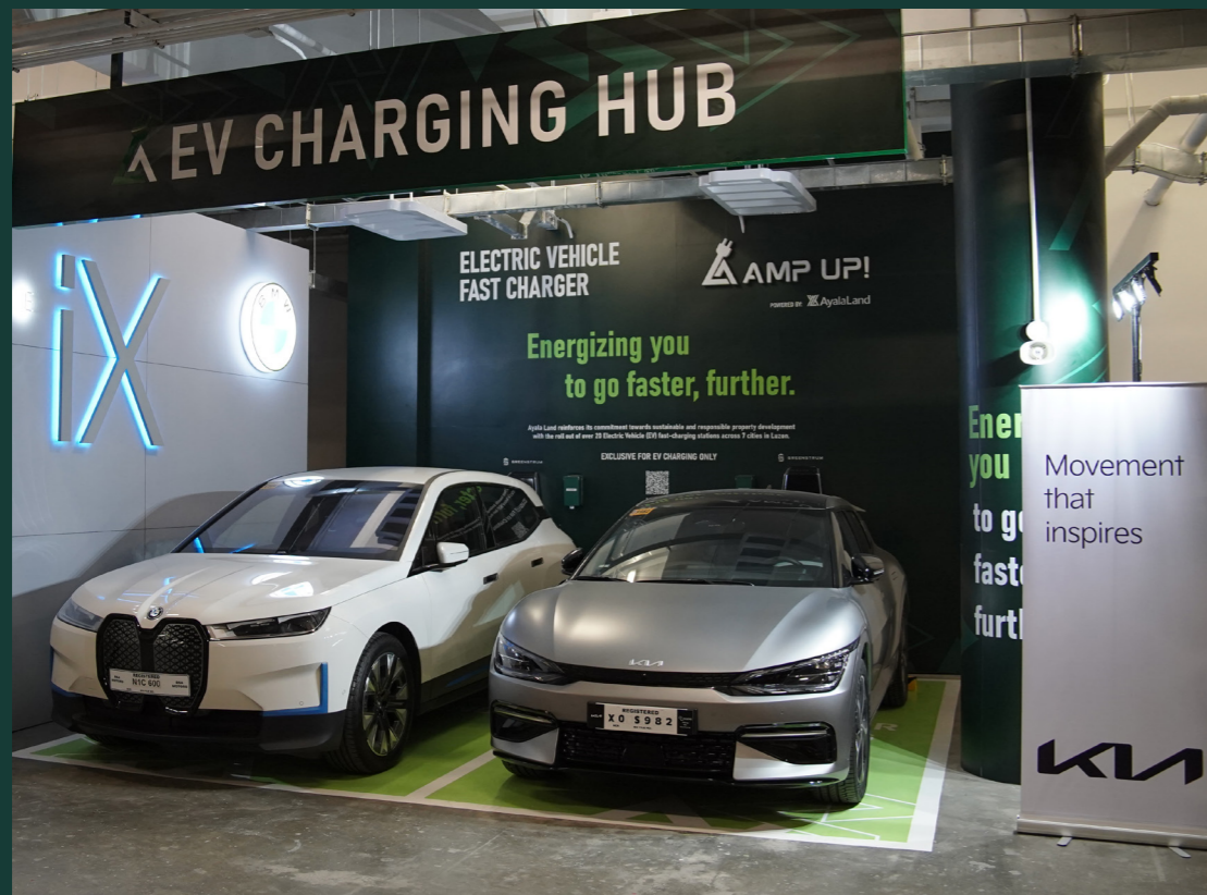
EV charging station in Ayala Triangle Gardens Tower Two
