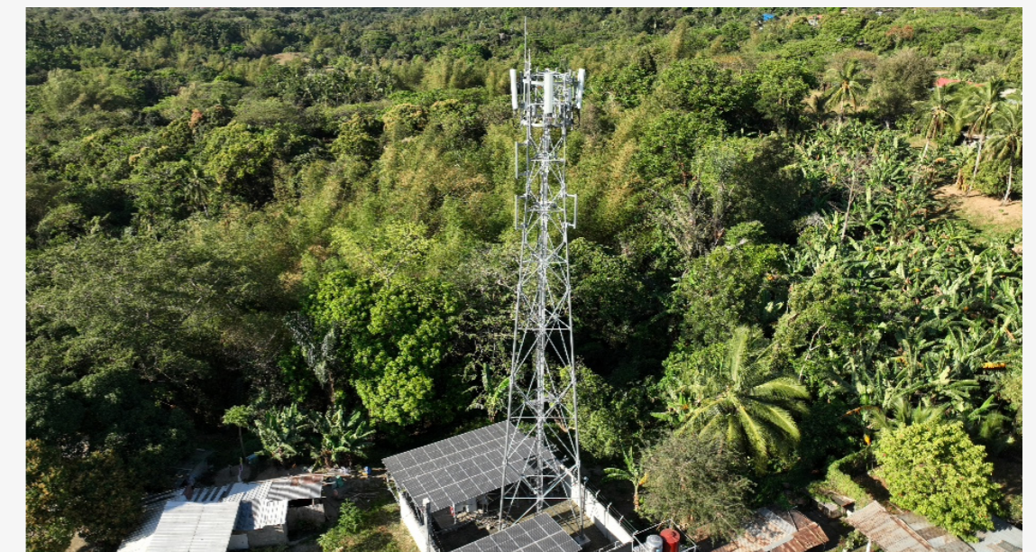
Globe piloted hybrid power alternative sources for cell towers in off-grid and bad-grid sites.
